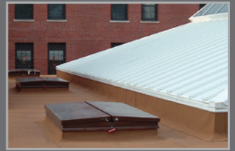
ROOF HATCH + SMOKE VENT
